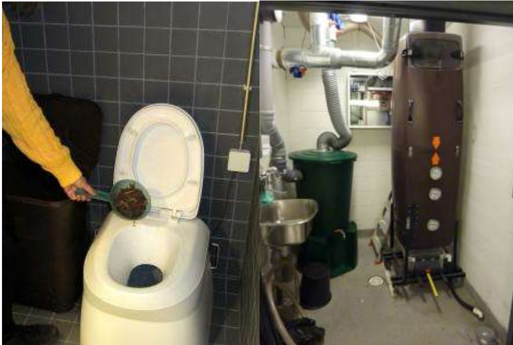
Figure 2. Two-story composting toilet seat in the first floor (left) and compost container in the basement (right).
