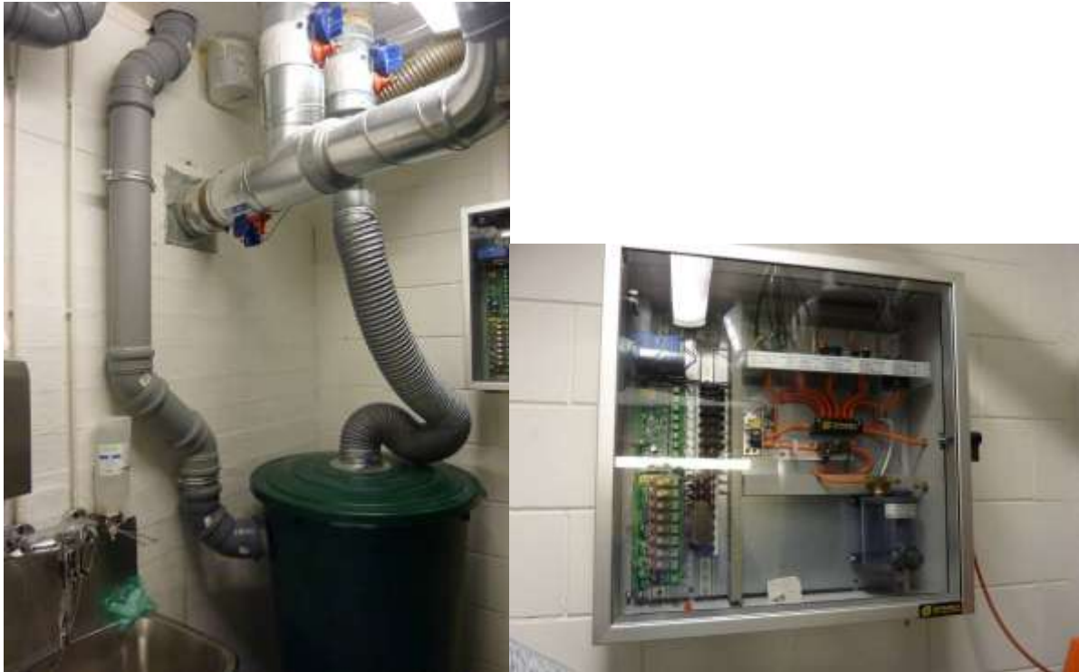
Figure 3. Urine tank and drain pipe from upstairs (left). In the same room is the gas monitoring system of the compost container of the two-story dry toilet (left).
