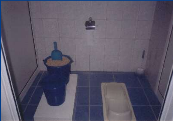
Squatting toilet with urine diversion
