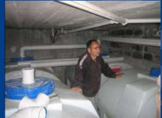
Urine storage tanks in the basement
