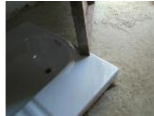
Door interfering with slab
