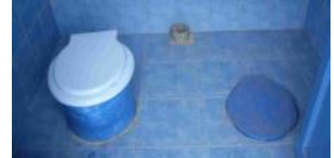
Poor ventilation design
