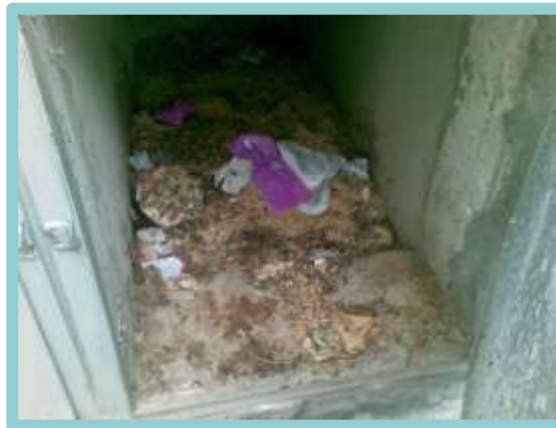
Too much sawdust added, also sanitary pads, toilet paper thrown inside toilet chamber
